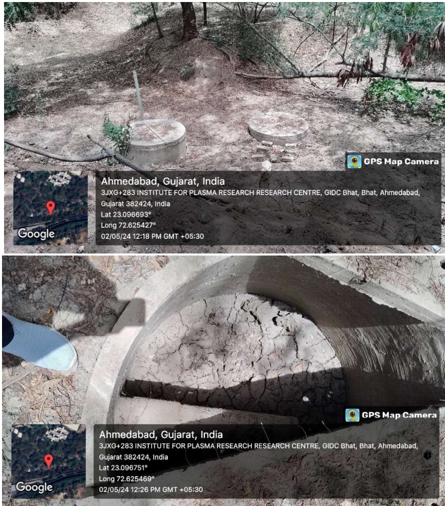
RWH system at IPR, Gandhinagar
