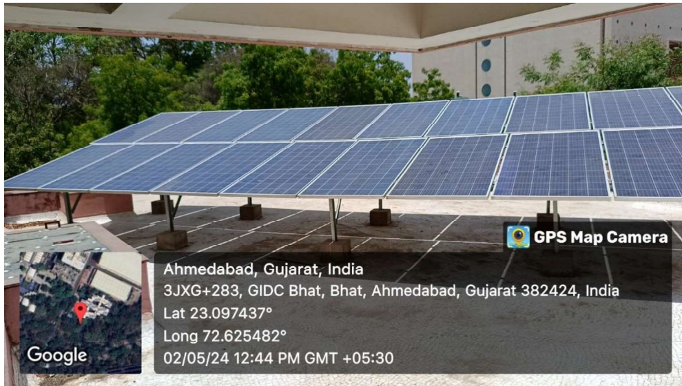
Solar Panel Installed on the roof of various buildings of IPR
