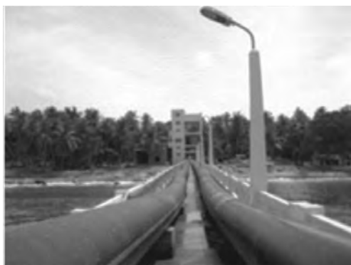
Desalination plant at Minicoy
