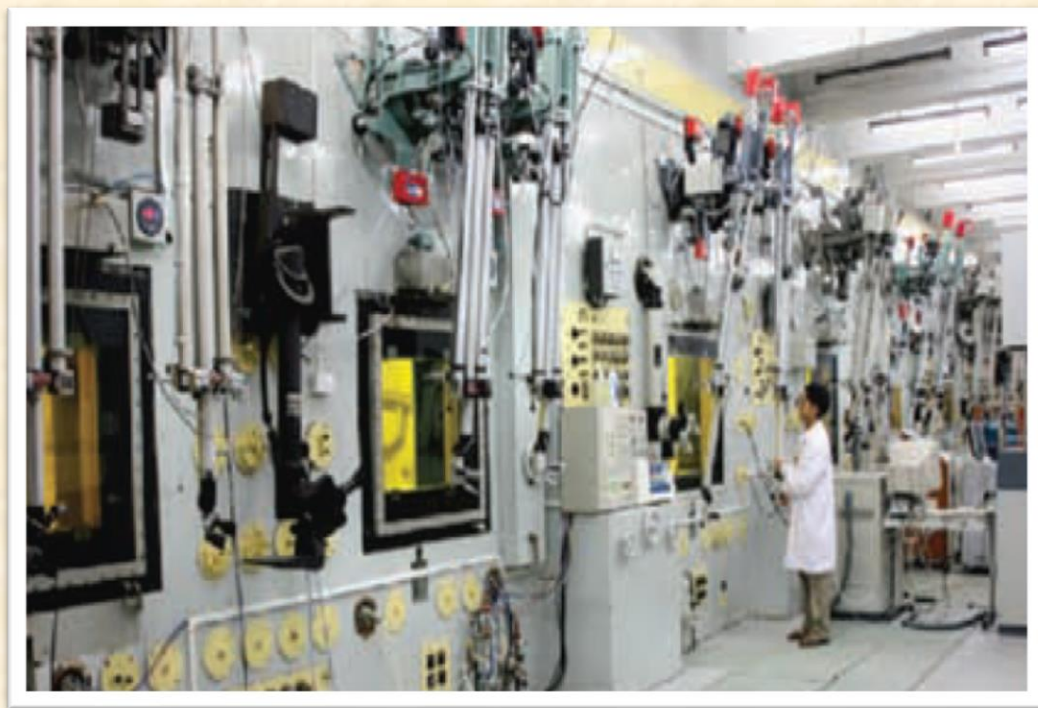
Hot cell facility for studies on radioactive materials at BARC
